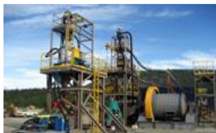
Lead Process Plant(Pb)
